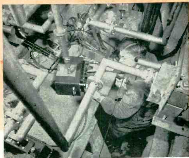
The Type 1601-A V-F-H Bridge set up to measure the antenna of WCBS-TV on the Chrysler Building, New York City. The antenna consists of 16 radiating elements. Measurements of the impedance variation of an individual element over the operating frequency band as well as impedance measurements of the whole array were made easily and accurately.
